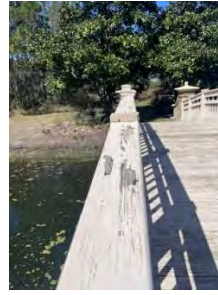
One of the missing caps
