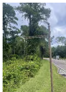
The Missing Bracket
